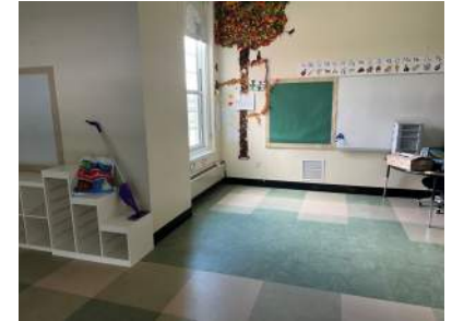
Perimeter FTR Heating
