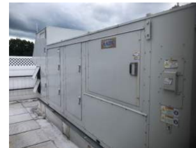
Rooftop Ventilation Unit
